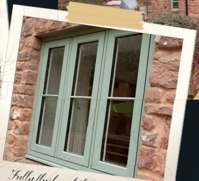
Timber windows in need of some TLC
